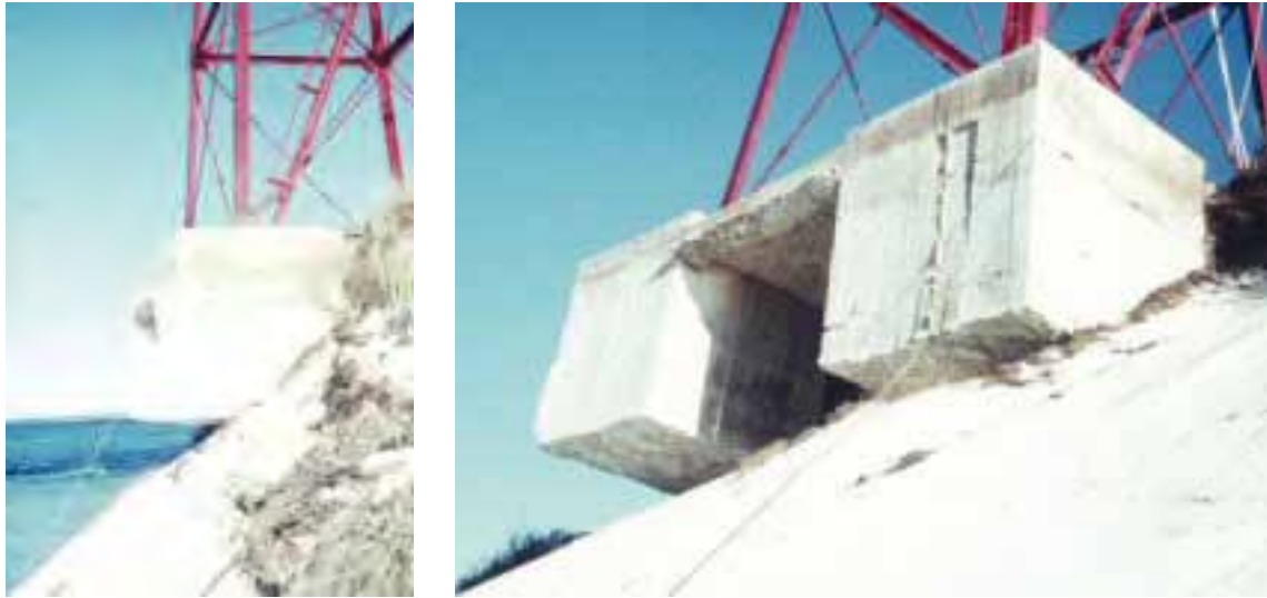
Figure 67. Fraser Island Light in the process of being undermined (Meakins Collection).
