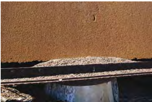
Figure 48. One of the few cement-filled barrels with evidence of timber staves. Note the severe corrosion around the base of the tank (Myra Stanbury).
