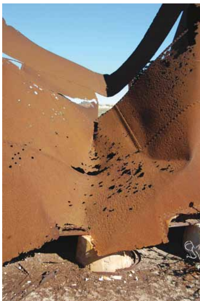
Figure 50. Collapsed wall of an oil storage tank (Myra Stanbury).
